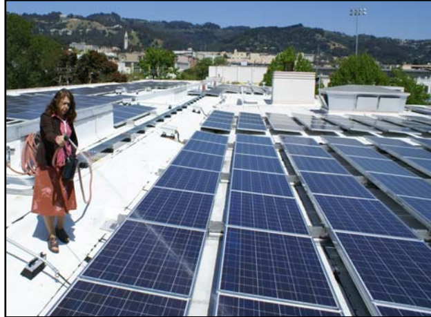
Washington Elementary is Berkeley's first solar school and Principal Rita Kimball goes the extra mile to insure maximum efficiency. The solar panels are expected to provide 70% of Wash
